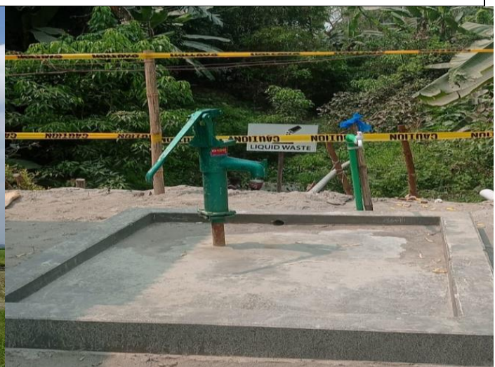
6. Tube well with protected base.
