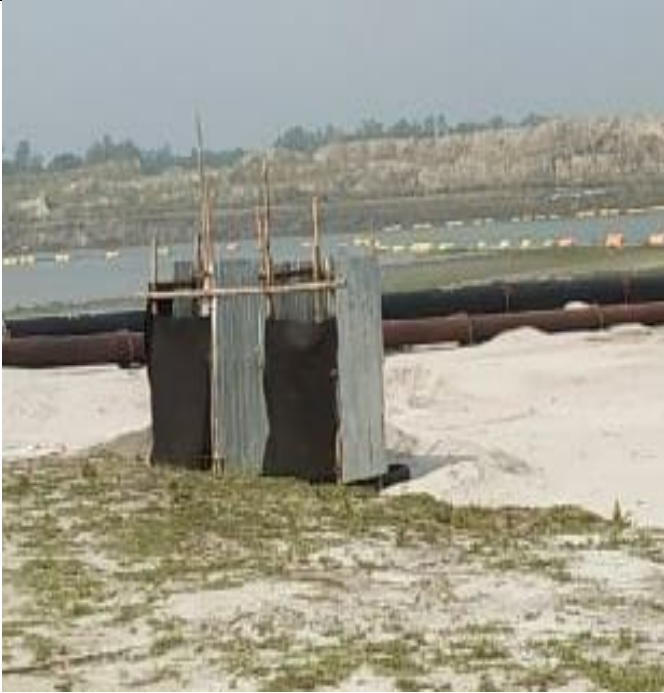
3. Unhygienic and inadequate toilets for labors.
