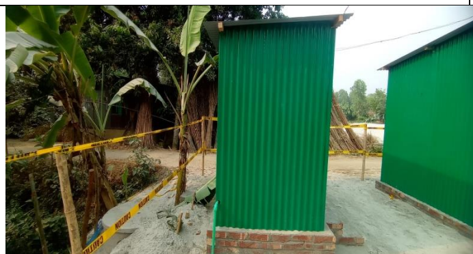
9. Toilet with sock pit.
